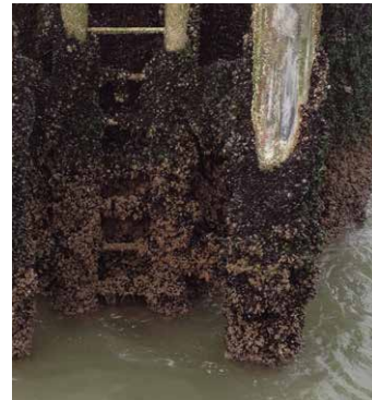
After several years the transition piece is completely covered with mussels and the ladder has disappeared amidst the growth.
